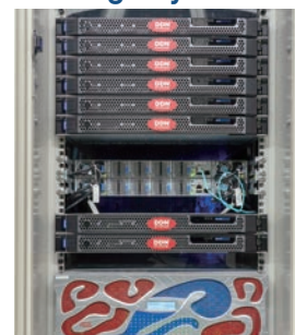
DataDirect Networks GRID Scaler file server system
