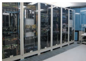
Network Operation Center
